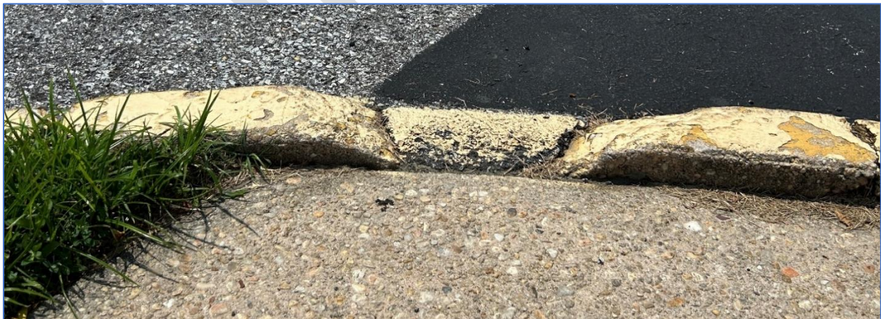
Inaccessible curb cut at the firehouse driveway intersection with 4 th Street
