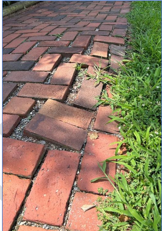
Issue found throughout the walk: brickwork in a poor state of maintenance
