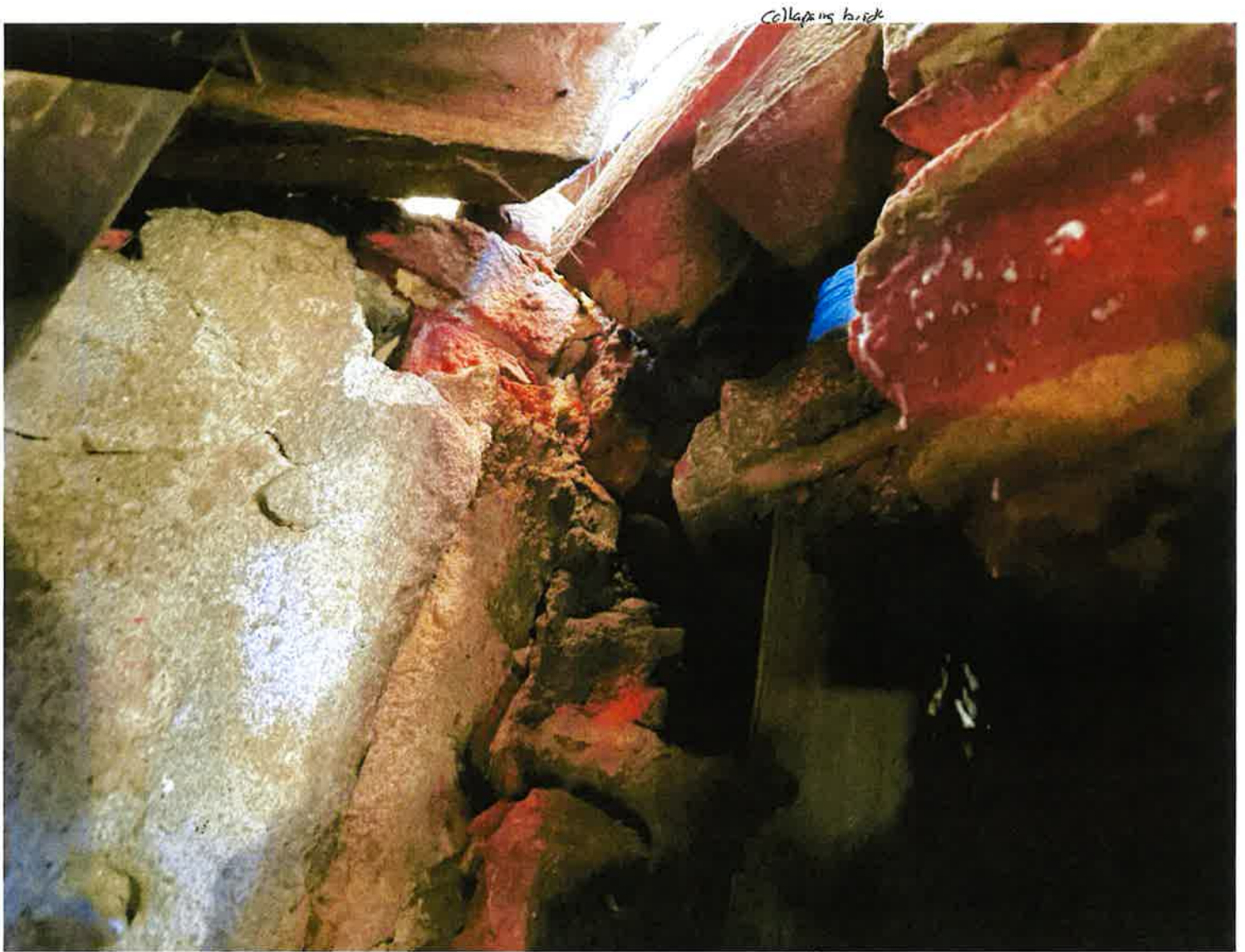
Crack extends to side wall of main
