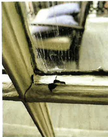
Flaking paint on a window
