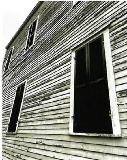
Flaking paint on a siding
