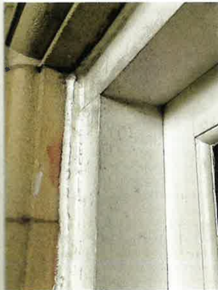
Mould on white paint.
