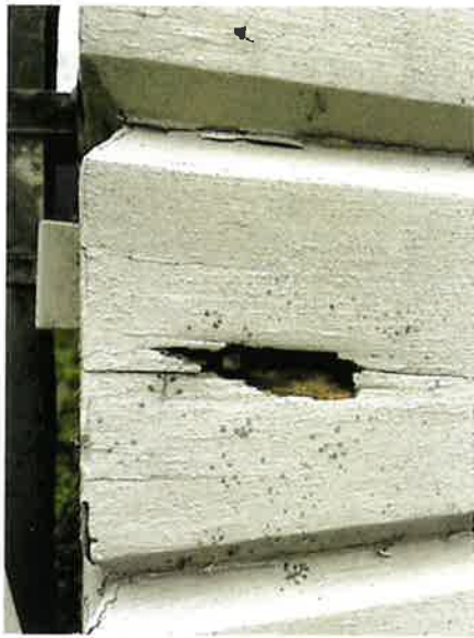
Rotted timber behind modern paint.
