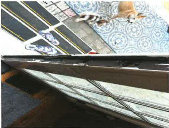
Reference pic for installers
